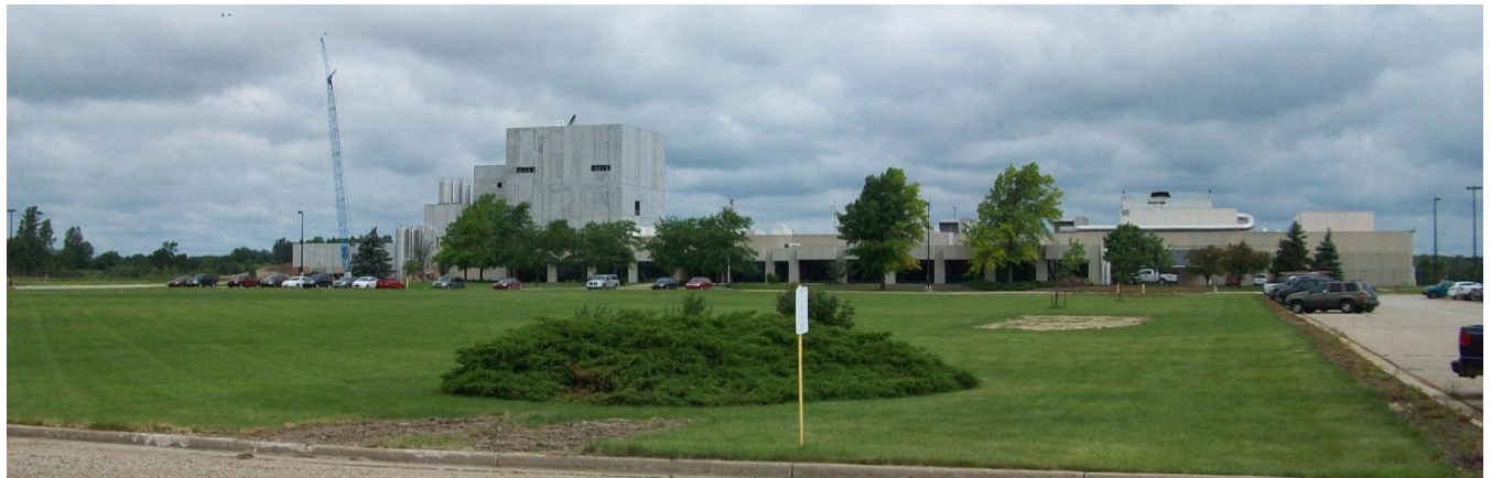
Construction at the old Delphi Coopersville plant as Continental Dairy prepares it for production.
